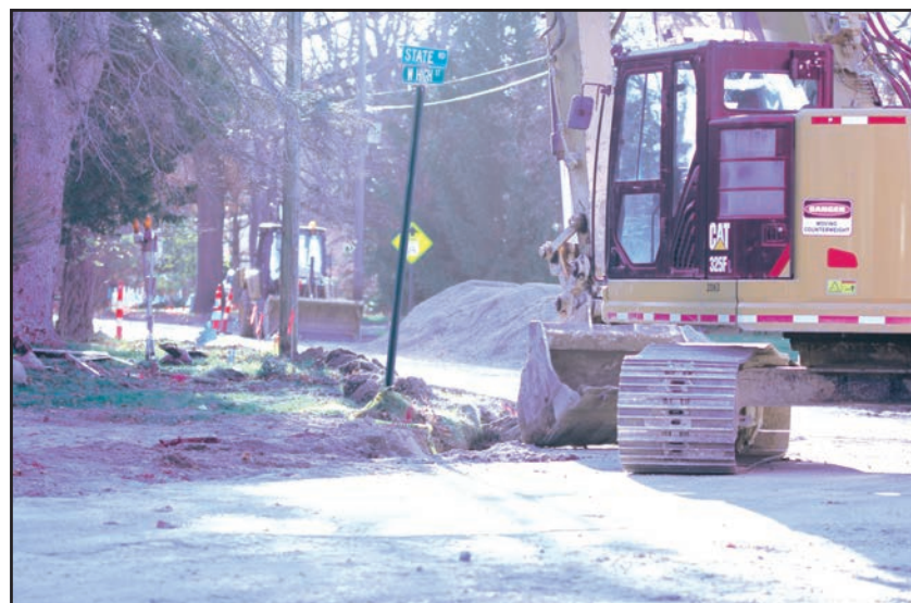
Construction workers hit a gas line at the intersection of W. High Street and State Road in Fenton on Monday, Nov. 13. Photo: Hannah Ball
