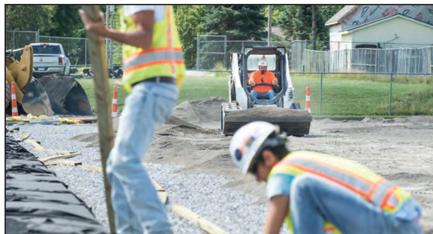
Brent Stevens and Christian Painter work on preparing the Lake Fenton High School track in early August before it was installed. Photo: Tim Jagielo
